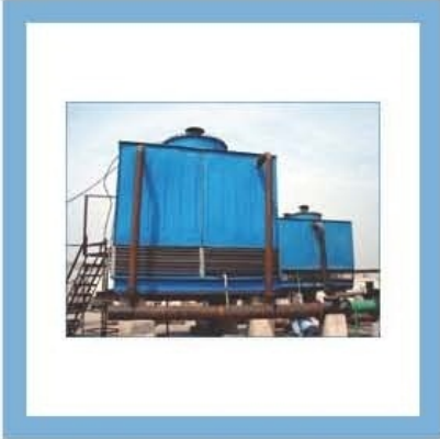
Induced FRP Cooling Towers
