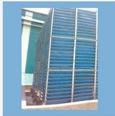
Natural Draft Cooling Tower
