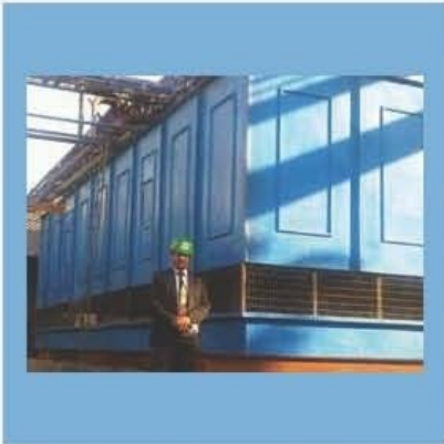
Induced Draft Cooling Tower
