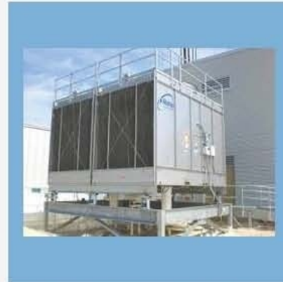
Water Cooling Towers
