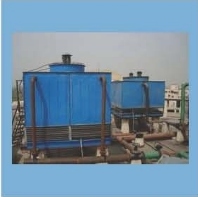
Heavy Industrial Cooling Towers
