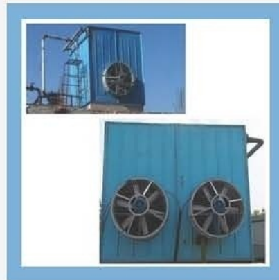
Forced Draft Cooling Tower
