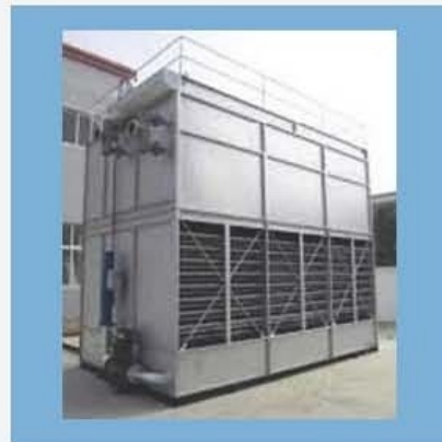
Cuboid Cooling Towers
