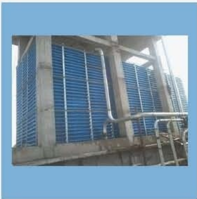
Jet Cooling Tower
